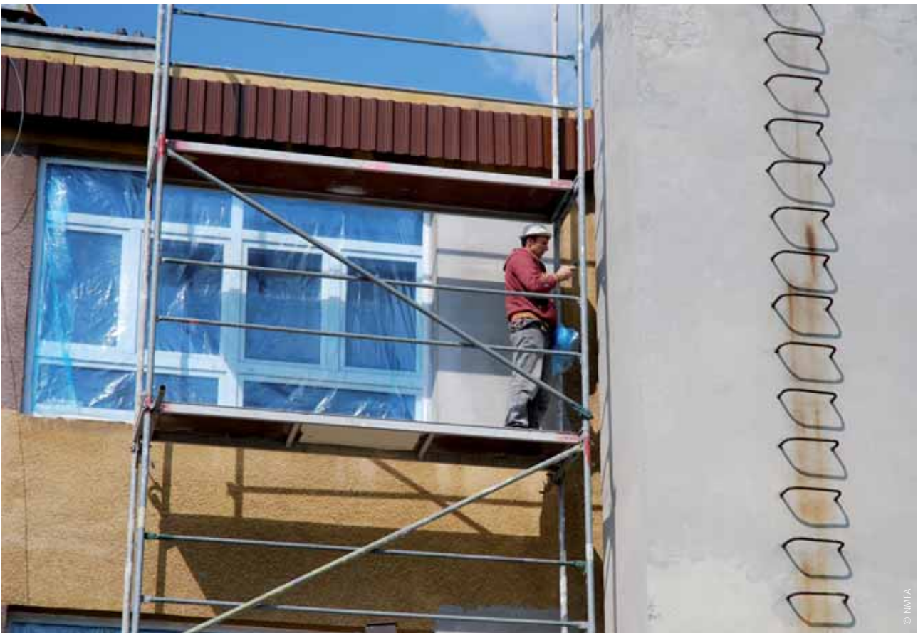
Improved thermal insulation in the Busko district in Poland has helped increase the energy efficiency of seven educational institutions.
