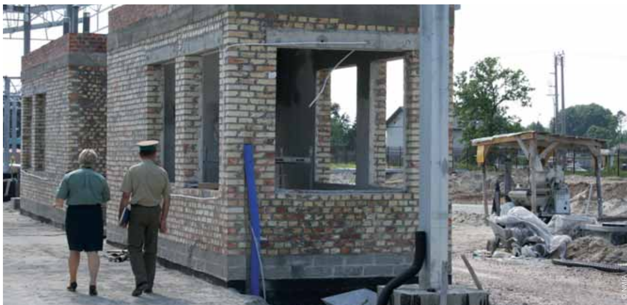
The modernisation of the Terespol border crossing at the Polish-Belarusian border at the edge of the Schengen area was one of the largest projects supported by the Norway Grants.
