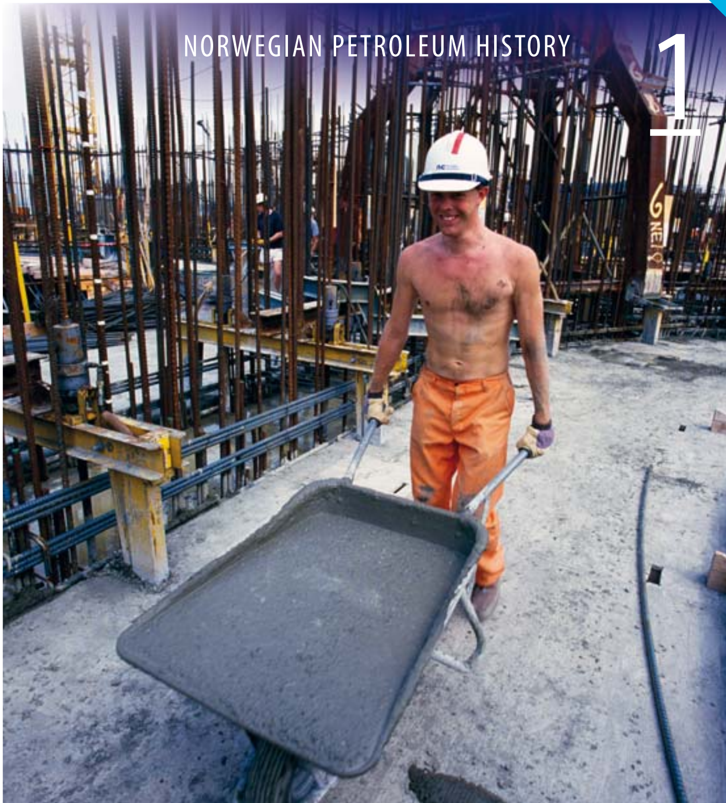
Pouring concrete for the foundations of the large concrete platforms from the 1980s was hard, physical work. (Photo: Leif Berge, Statoil)
