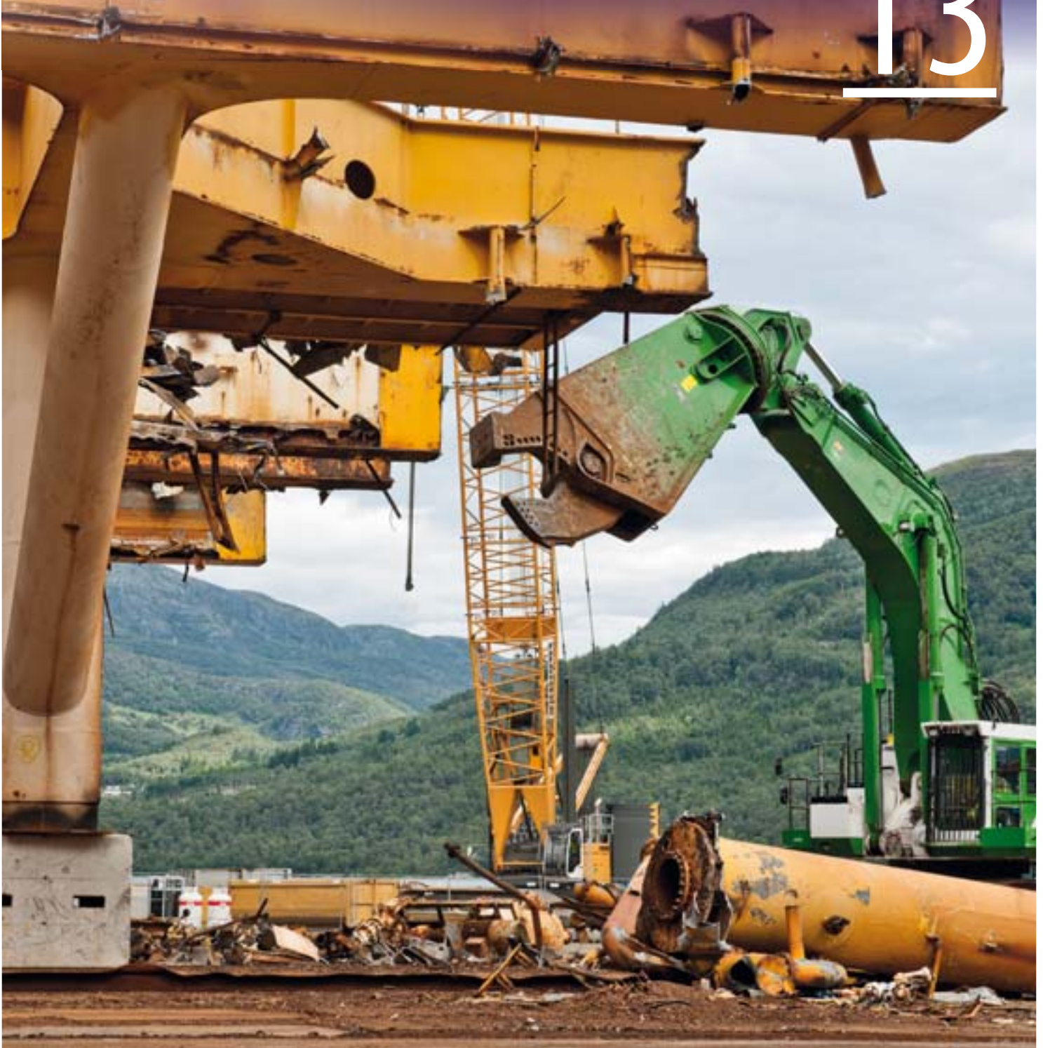
The Norwegian shelf has matured, and the first installations are being removed and scrapped on land. (Photo: Monica Larsen, NPD)
