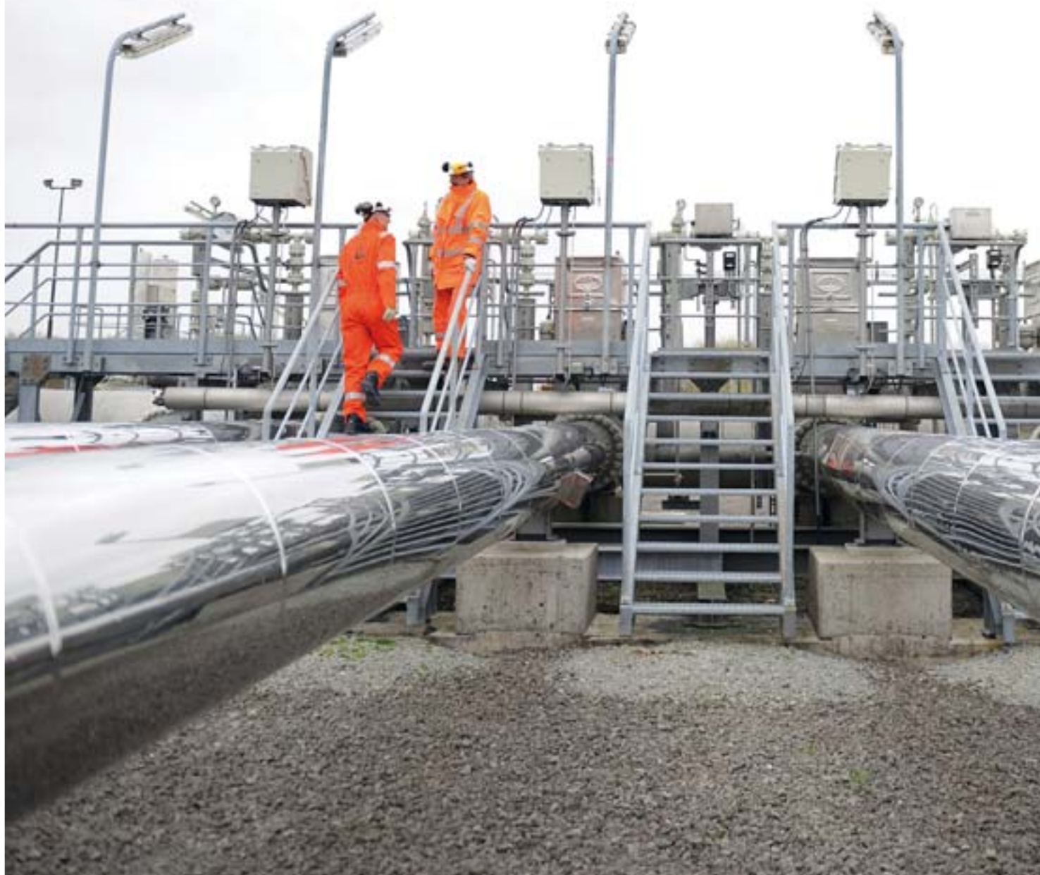
Norwegian export gas arriving at the terminal in Emden, Germany. The Norwegian Petroleum Directorate makes sure that the measuring instruments work precisely. (Photo: Emilie Ashley, NPD)
