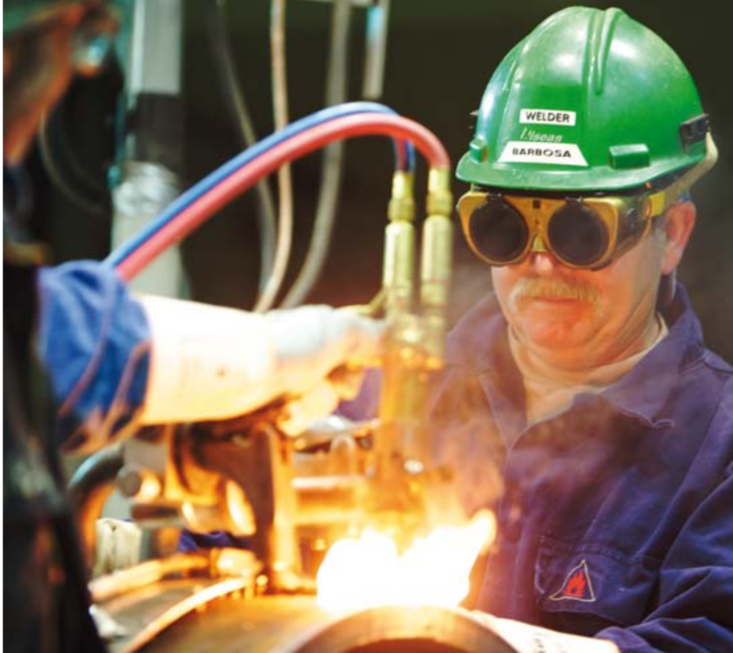
The welding seams must be extremely precise when laying pipeline on the Norwegian shelf. (Photo: Anette Westgaard, Statoil)
