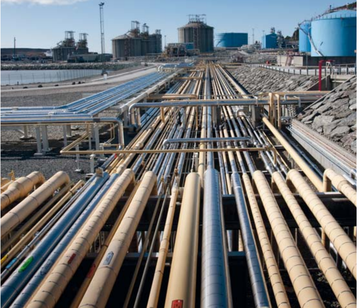
Gassco's gas treatment facility at Kårstø is a hub for Norwegian gas export. (Photo: Øyvind Hagen, Statoil)
