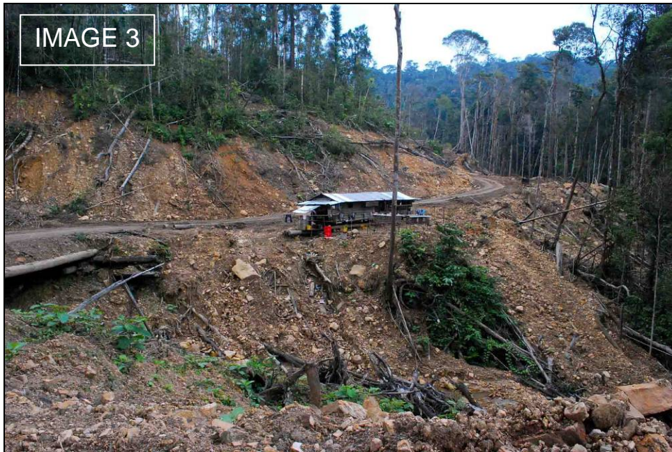
Figure 17: Forest cleared in excess of limits, no buffer zone left alongside stream (the stream is just outside the picture, in the slope in the foreground). The stream clogged with logging debris can be seen towards the bottom of the picture. See Figure 12 for location.
