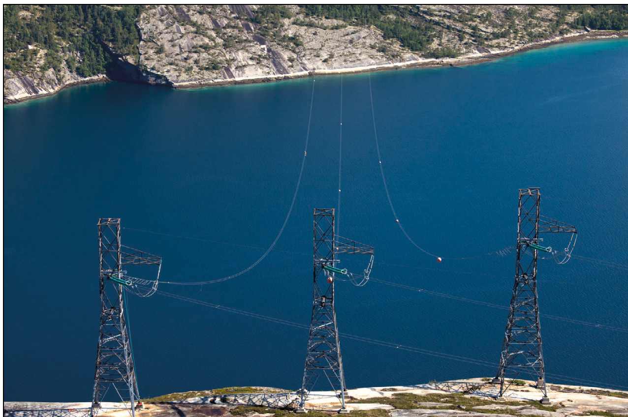
Figure 6.1 Through Statnett, the state owns the majority of the central electricity transmission grid in Norway.
