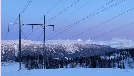
Photo: Statnett SF
